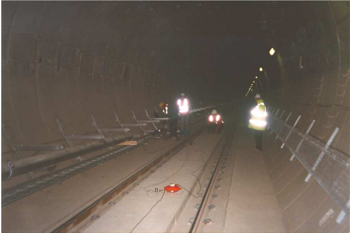
Figure 6.4: Photograph of the tunnel, showing at left the supports for the incomplete track-side walkway and above them the wedge-shaped keys in the tunnel lining. The accelerometers are set out along the floating-slab track and the rest of the equipment can be seen in the background.
