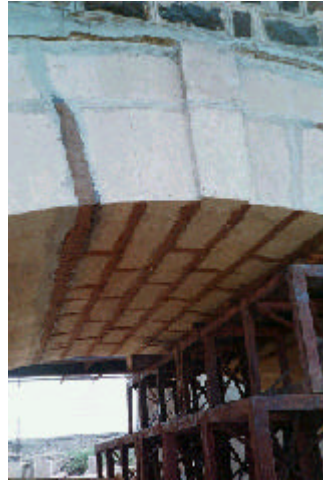
Fig.3 Crown stones of the arch opened up due to abutment movement
