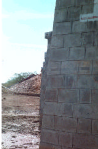
Fig.2 Piers of plate girder bridge suffered rotation
