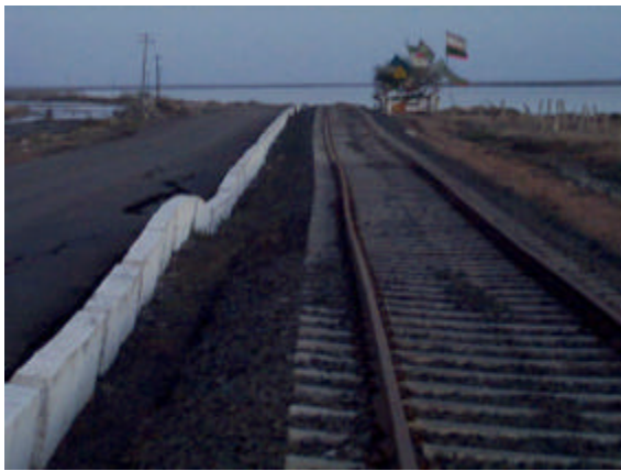
Figure 12 Lateral spreading at Navalakhi port.
