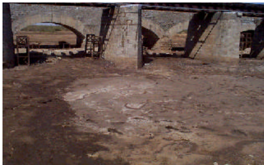
Fig.1 Liquefied bridge site during Bhuj earthquake of 2001
