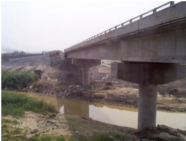
Figure 2 : Nantou New bridge after the 1999 Ji-Ji earthquake showing arrangement of piers relative to the river.
