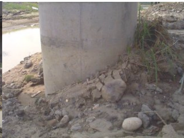
Figure 3 : Nantou new bridge pier after the Ji-Ji earthquake showing build-up of soil on the upslope face and gap downslope.
